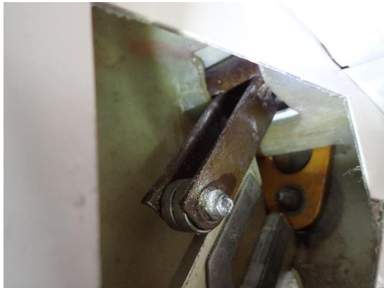
Image 3 Disconnected elevator control
